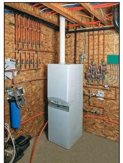
Baxi Luna HT 1.33 condensing boiler atop the Modulo storage tank.
